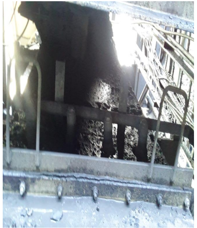
DSS sprinklers at BC-01 Tail end
