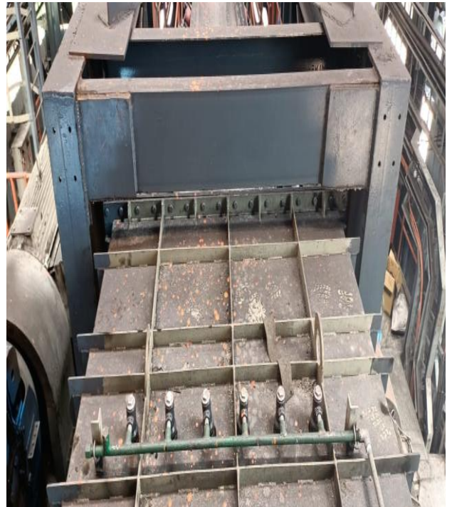
DSS sprinklers at PC Head end
