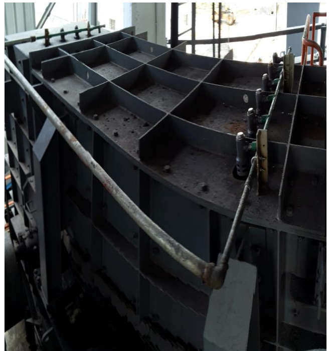
DSS sprinklers at Apron Feeder
