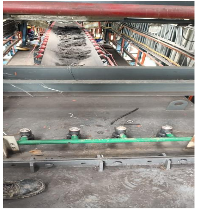
DSS sprinklers at BC-02 Head end
